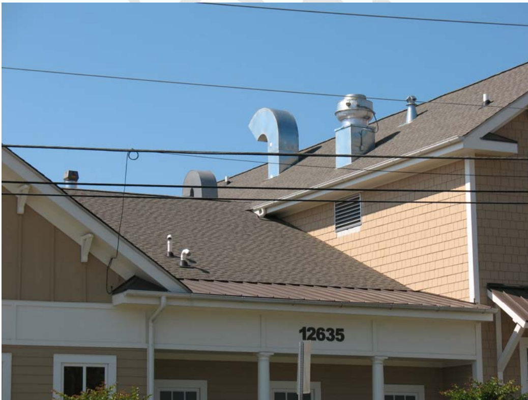
PICTURE #2: ROOFTOP VENTILATION SYSTEM AS SEEN LOOKING NORTH ON CRABAPPLE ROAD
